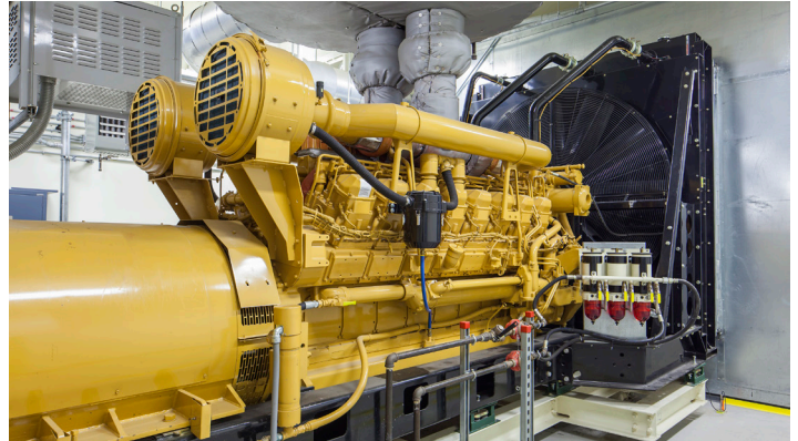
A permanent diesel generator, shown above, is a reliable backup option for larger businesses during a power outage.
